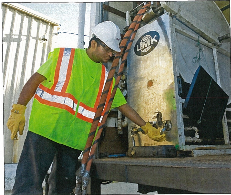
Santos Romero, equipment operator, works with the steam hose reel used in the company's sewer lateral rehabilitation system from LMK Enterprises.
